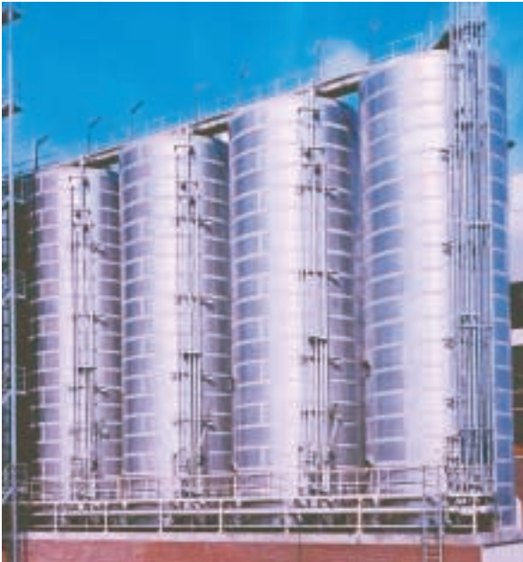
Beer is fermented, deep-cooled and stored in vertical tanks at temperatures of -1 °C and over, depending on the type of beer, with an accuracy of +/- 0.1 degrees.
