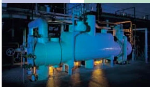
Chemical plant for chlorine liquefaction.
