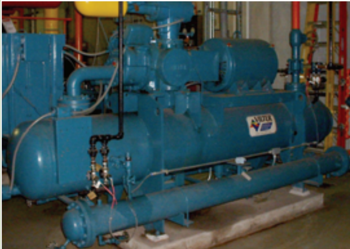
Compressors for refrigeration system in machine room with ammonia detection and alarms
