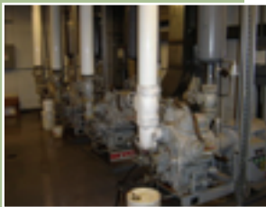
Room requiring ammonia detection
