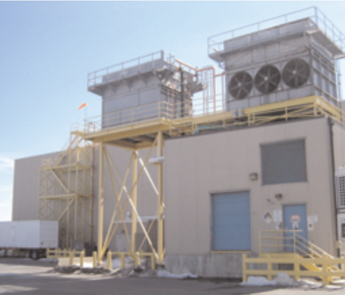
Detached building with condenser
