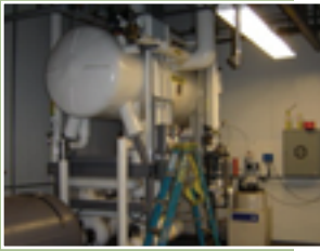
Ammonia expansion tank in machine room with ammonia detection and alarms
